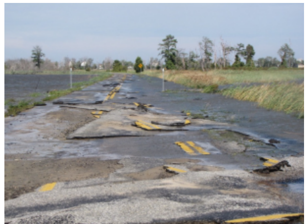
Figure 8. A road damaged by flooding from Hurricane Irene at Prime Hook National Wildlife Refuge.
