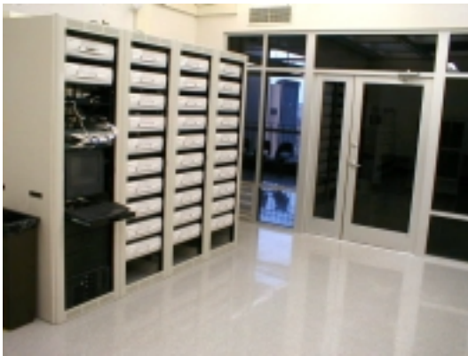
Figure 6: Overall view of PC Room
