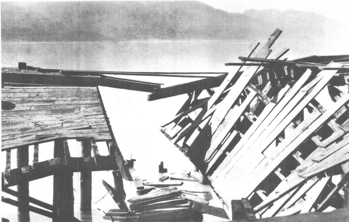
7.—Dock failure in late 1920's. Note that failed section has tipped shoreward. Photograph courtesy of James Derringer.
