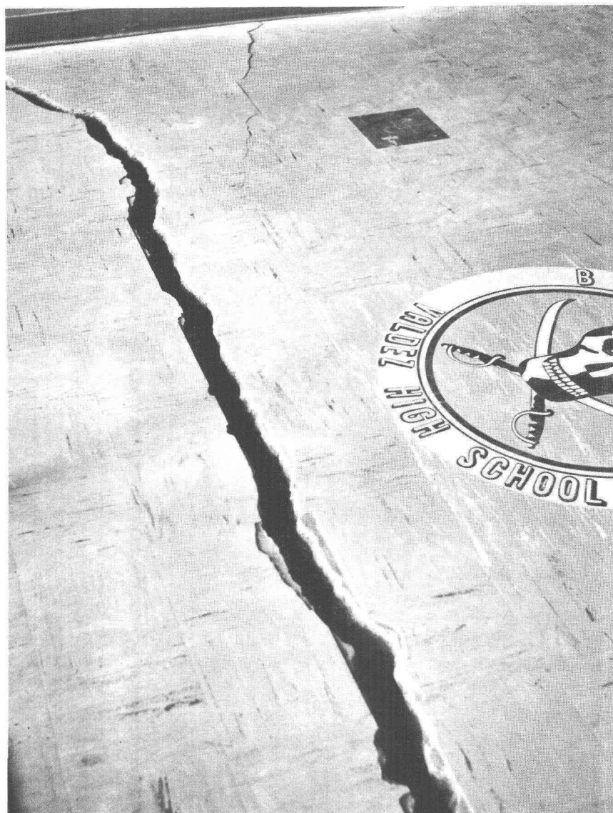
19.—Transverse fissure through the concrete foundation slab of the Valdez High School, Sherman Street and Empire Avenue.
