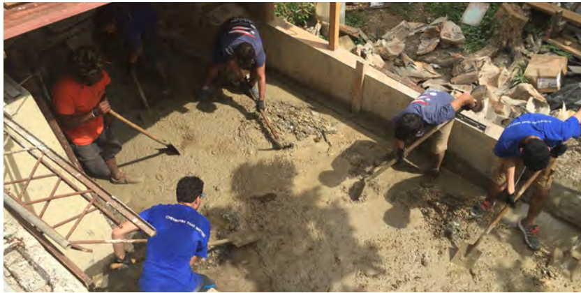
Students mixed and shoveled concrete in order to help build a roof.
